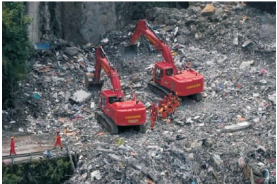
areas within a kilometer radius of the disaster site, relocating over 1,100 people, Chongqing authorities
